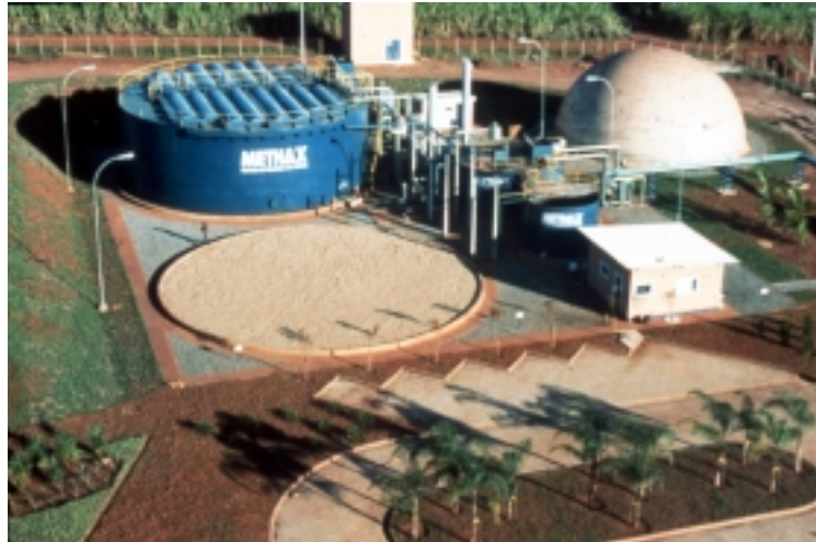
A digester treating dilute wastewater at a fuel ethanol production plant in Brazil (photo credit: Paques BV)
